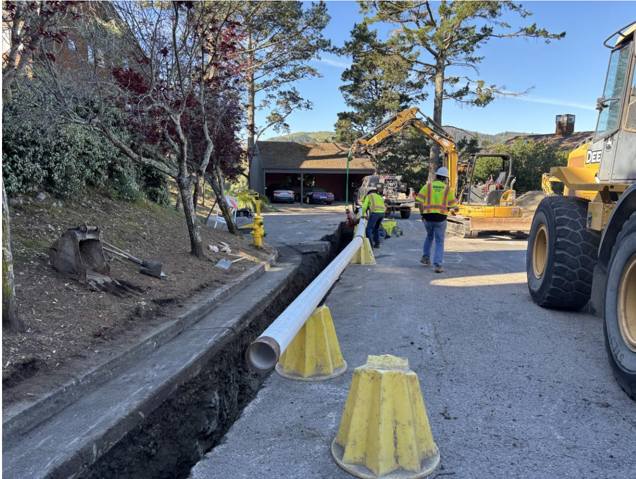
Installation of seismically resilient welded steel pipe during Marin City Phase 2 construction.
